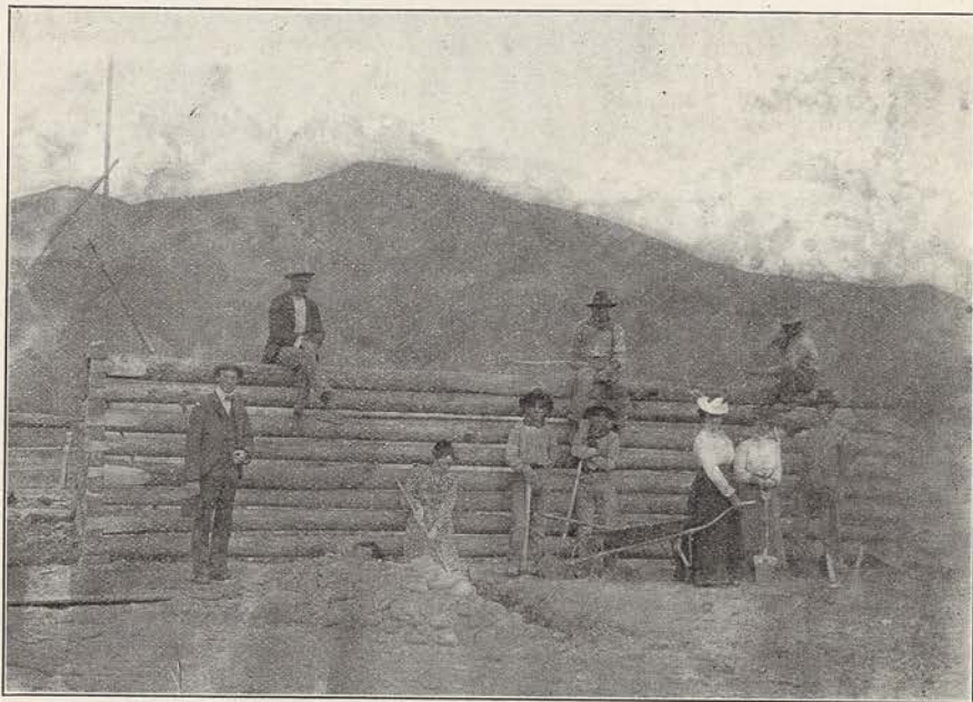
BEGINNING WORK ON THE MISSION HOUSE, OCTOBER, 1901 Miss Stockdell holds the shovel; the other two women are teachers in the government school
