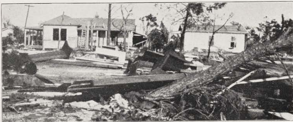
SHOWING THE WRECKAGE AROUND ST. CUTHBERT'S CHURCH, BOYNTON, FLORIDA In the foreground are bits of flooring on the site of the church but nothing else remains to indicate a place well loved by a loyal colored congregation
