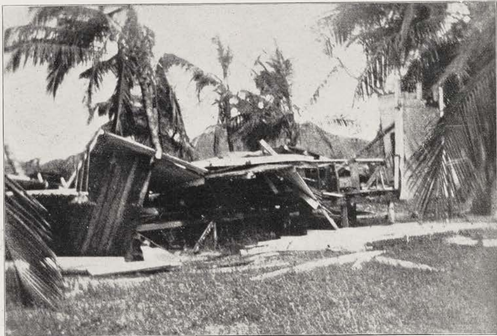
THE NEW WORLD SCHOOL, PORTO RICO, REDUCED TO KINDLING Wind was still shrieking through the trees when this photograph was made. It well represents the meaning of the words "totally destroyed" as used by Bishop Colmore
