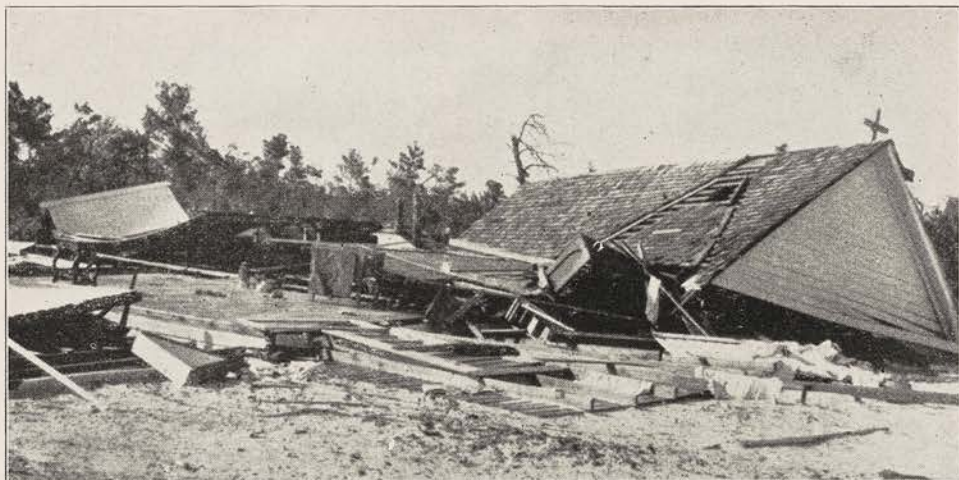
CHAPELS WERE LIFTED BODILY INTO THE AIR BY THE FORCE OF THE HURRICANE
