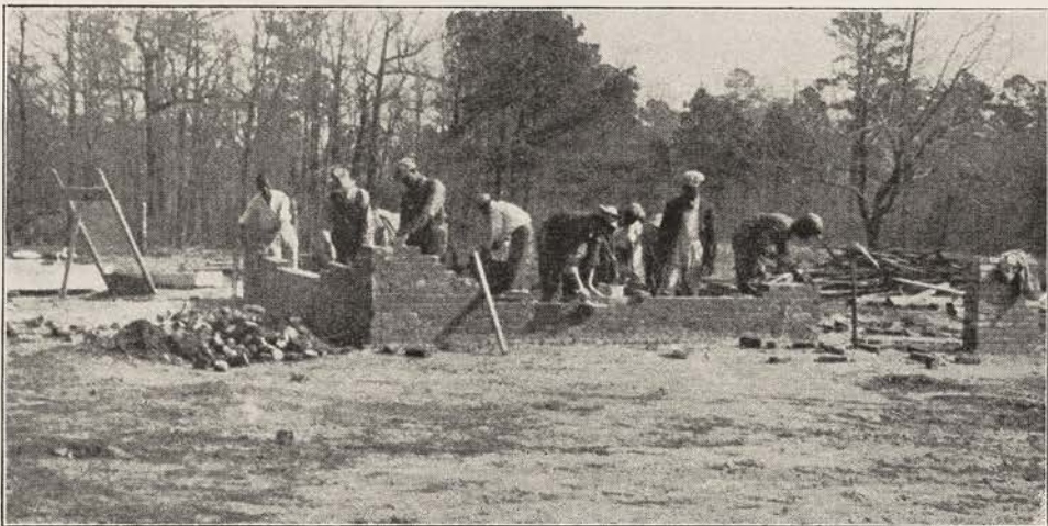
A CLASS IN MASONRY, VOORHEES NORMAL AND INDUSTRIAL SCHOOL Bricklaying is one of the seven trades taught to boys in an effort to fit them for lives of Christian usefulness in their communities. Voorhees also provides three different industrial courses for girls
