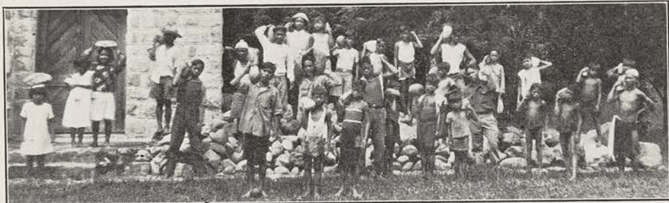
CARRYING STONES FOR A NEW ALL SAINTS' MISSION, BONTOC, P. I. Boys and girls of All Saints' School collect the materials for a new building made possible by a $6,000 gift from the Diocese of Rhode Island
