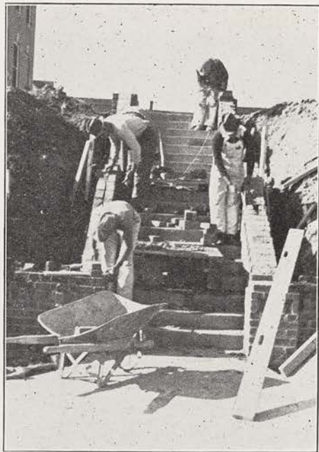
FUTURE BRICKLAYERS Students at St. Paul's School, Lawrenceville, Virginia, learn useful trades through doing the actual work involved
