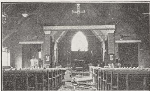
WRECKED INTERIOR (above) of Our Saviour Church, erected entirely by the congregation itself.
